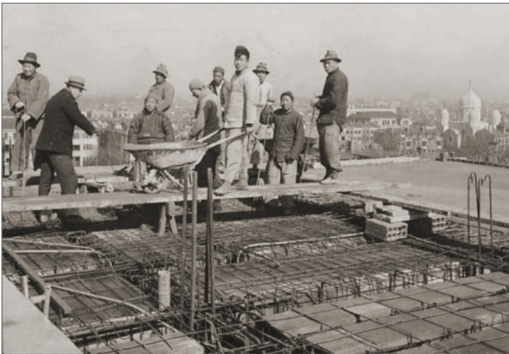
Figure 9: A. V. Kooklin (left) and workers on the roof of Hanray Mansions; the Orthodox Cathedral is on the right. Kooklin family archive
