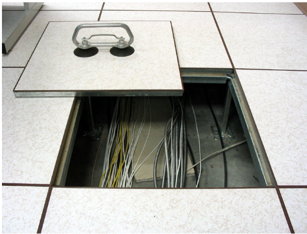
Figure 2.3: A raised floor creates a hidden void for the passage of cables.
